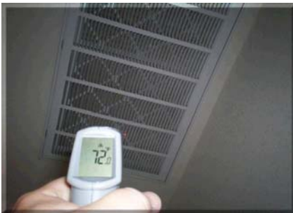
Photo: 2. View of AC inlet temp (1)
