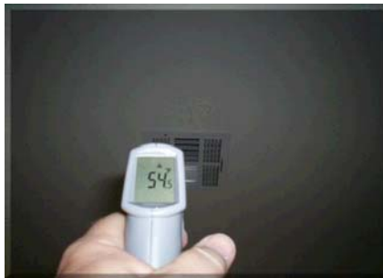
Photo: 2. View of AC outlet temp (1)
