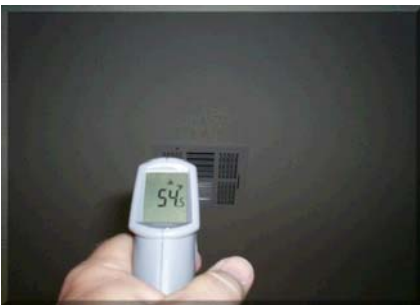
Photo: 2. View of AC outlet temp (1)
