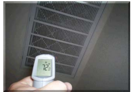
Photo: 2. View of AC inlet temp (1)
